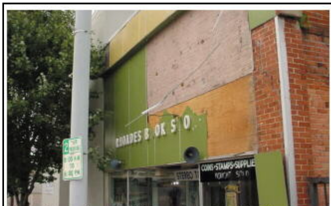
The facade of Rhoades Book Store on Ninth Street was partially torn off during the storm.
